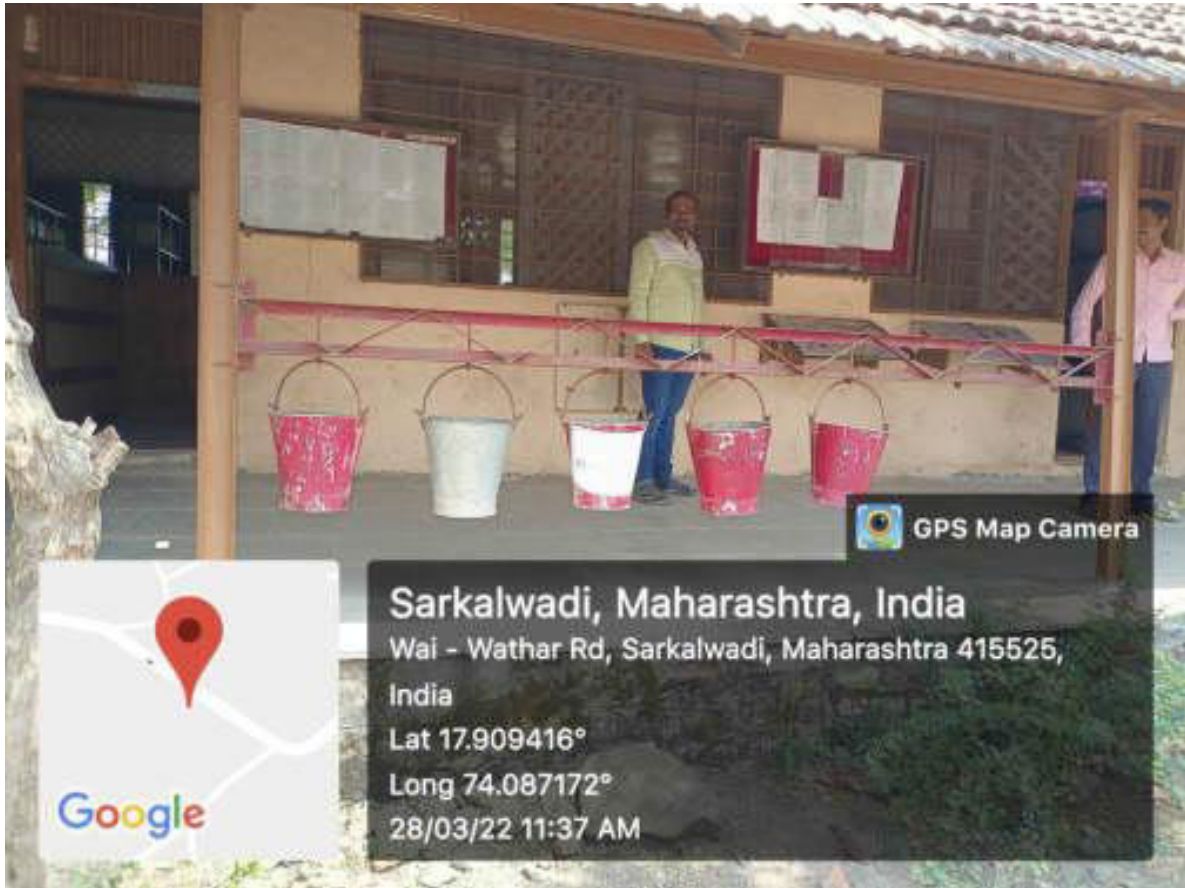
Fire Extinguishing System
